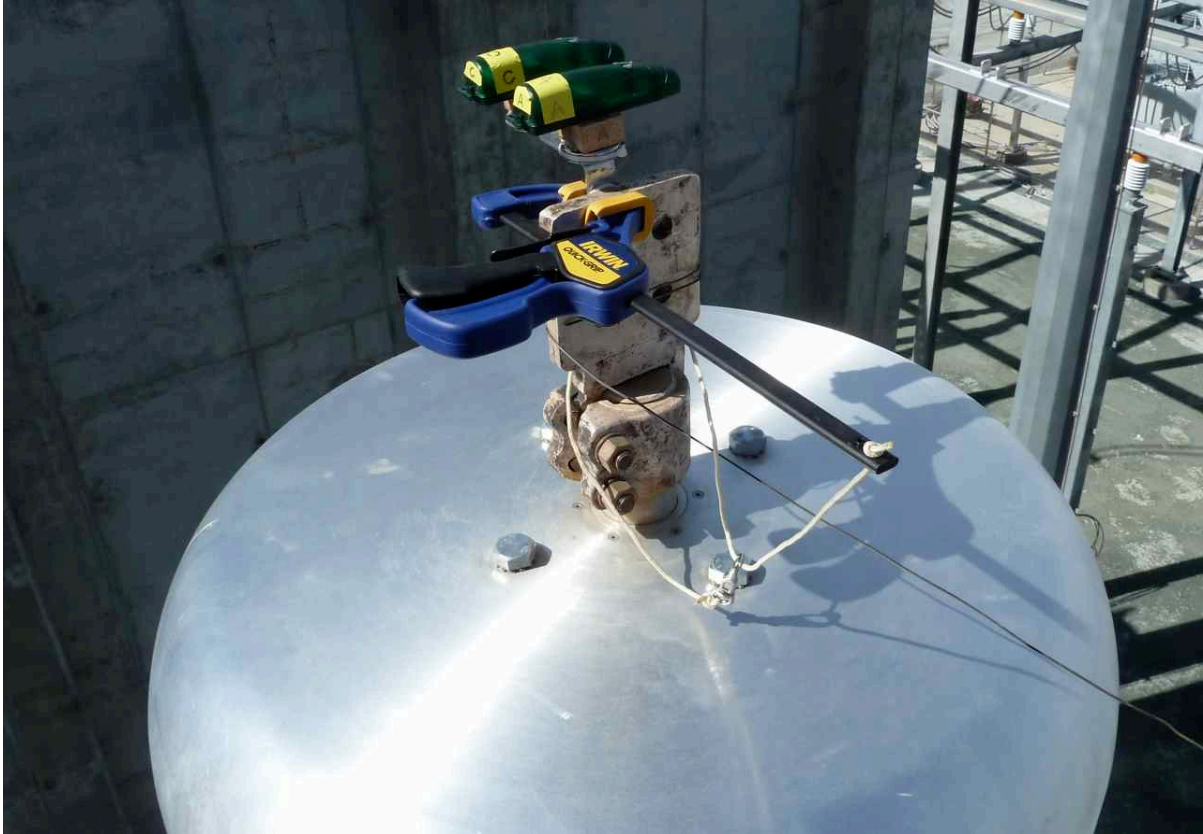
Figure 6-2 Accelerometers attached to bushing terminal post
