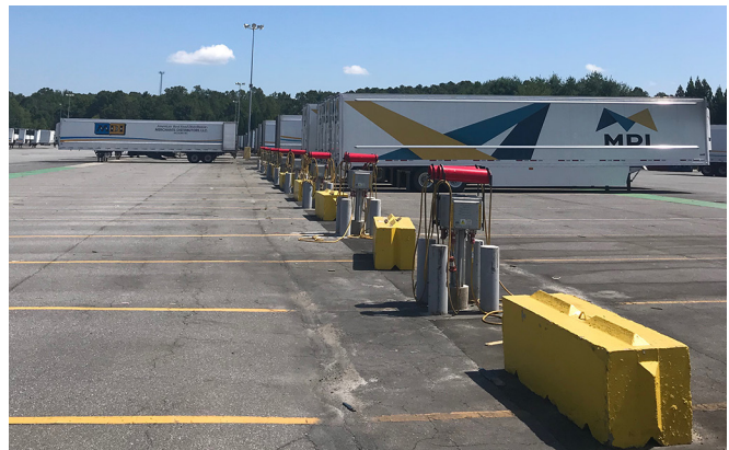
Trailers operating on 480-volt electric service points in the staging area (during the daytime when most are out for deliveries).
