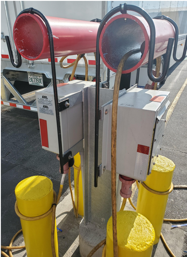
MDI installed 36 electric service points, enough to support more than 100 eTRUs.
