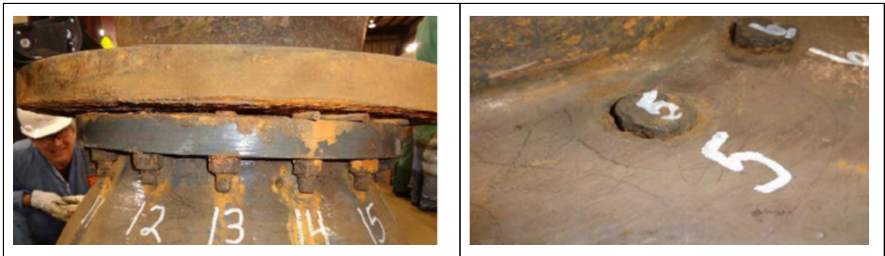
Figure J-6 Gap between bottom column and suction bell flange
