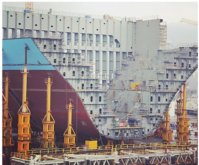
Figure 2. Modular construction. Modular construction is the industry standard for shipyard-based fabrication and assembly. Shown here is a Maersk Triple-E class vessel under construction, at the DSME shipyard in Okpo, South Korea. Used with permission according to Creative Commons terms. By Maersk Line - Flickr photo page, CC BY-SA 2.0, https://commons.wikimedia.org/w/index.php?curid=27646189 .
