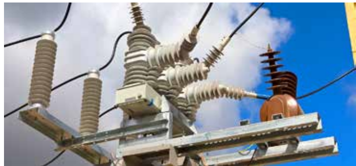
Figure 1 – Some modern protection devices have advanced features to reduce damage to distribution assets, minimize energy into a fault during reclose attempts, and save fuses to reduce the work of field crews.
