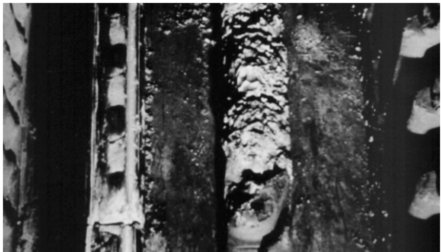
Figure 2 – Closeup of the damage
