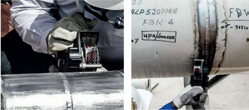
Figure 2-24 Photographs showing general use of bristle-blasting tool to remove surface scale and coatings
