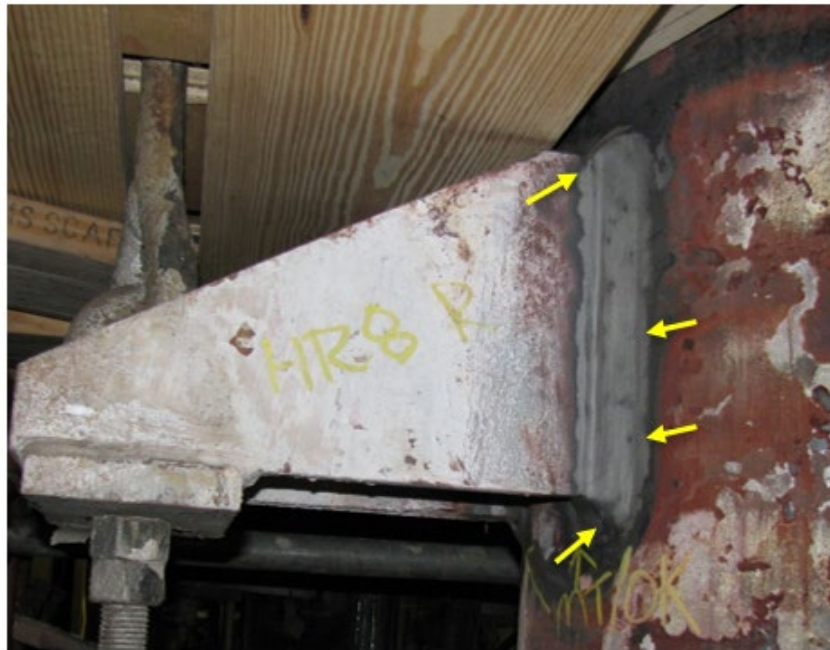
Figure 2-22 Incomplete surface scale removal from hanger attachment lugs, which could lead to false/missed indications
