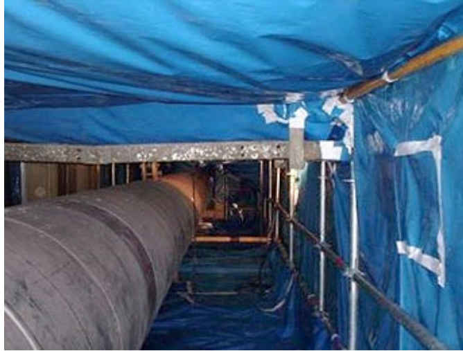
Figure 2-30 Example of insulation abatement/sandblasting enclosure around a hot reheat piping system after blast media removal
