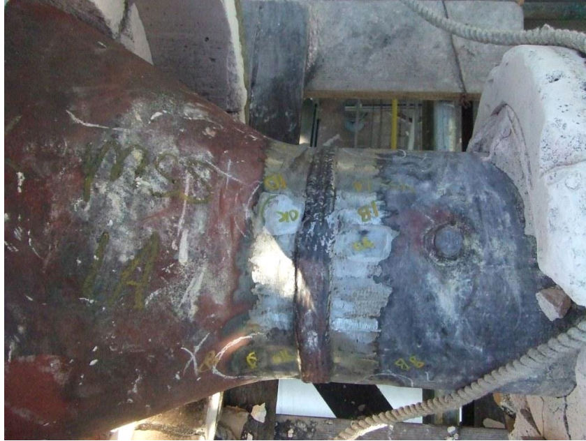
Figure B-7 Girth weld: example of incomplete oxide removal from the weld beads
