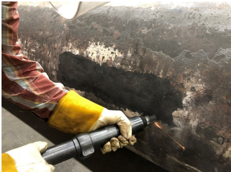
Figure 2-25 Example of high-temperature scale removal from a seam weld using a pneumatic needle descaler
