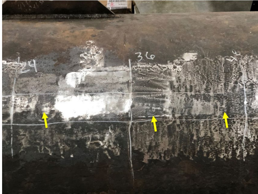
Figure 2-21 Incomplete surface scale removal along a long seam weld by power grinding. This surface condition is unacceptable for most NDE methods.
