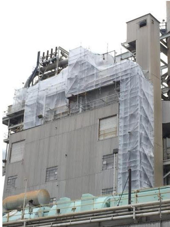
Figure 2-31 Example of insulation abatement/sandblasting enclosure built around scaffolding during a high-energy piping inspection
