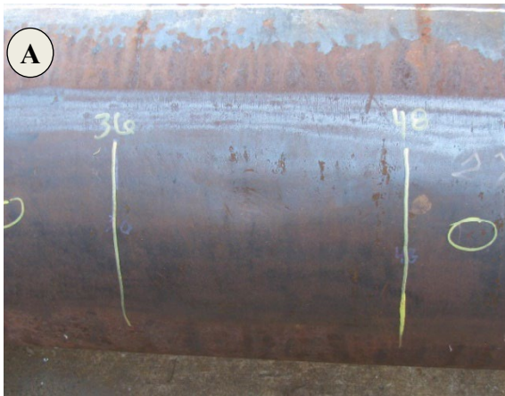
Bad manual grinding/sanding preparation; mill scale left on surface
