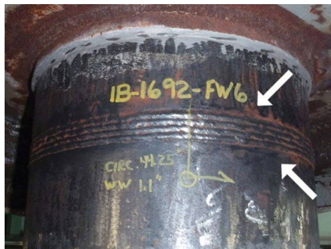
Figure 2-18 Improper surface scale removal by power wire brushing
