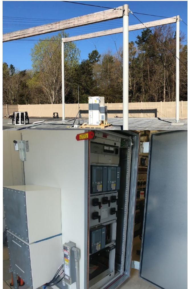
Figure 6. The IEC 61850-based protection and control system hardened against E1 HEMP (Top: the full system deployed, which includes a shielded protection and control module in the substation control building and merging units housed in shielded enclosures inside circuit breaker control cabinets. The merging units and protective relays housed inside the shielded protection and control module are connected by fiberoptic cables. Middle: the protection and control module being tested up to 50 kV/m in EPRI's MIL-STD-461G/RS105 guided wave test facility in Charlotte. Bottom: the protection and control module deployed inside a substation control building.)
