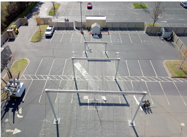
Figure 5. EPRI's outdoor MIL-STD-461G/RS105 test facility in Charlotte, North Carolina (Electronic devices, such as DPRs, are subjected to E1 HEMP pulses up to 50 kV/m to determine the level of insult that causes damage or disruption.)
