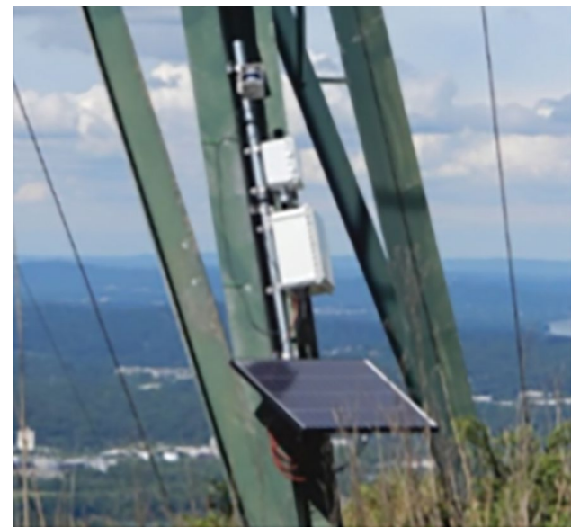
LineVision system as deployed in the field
