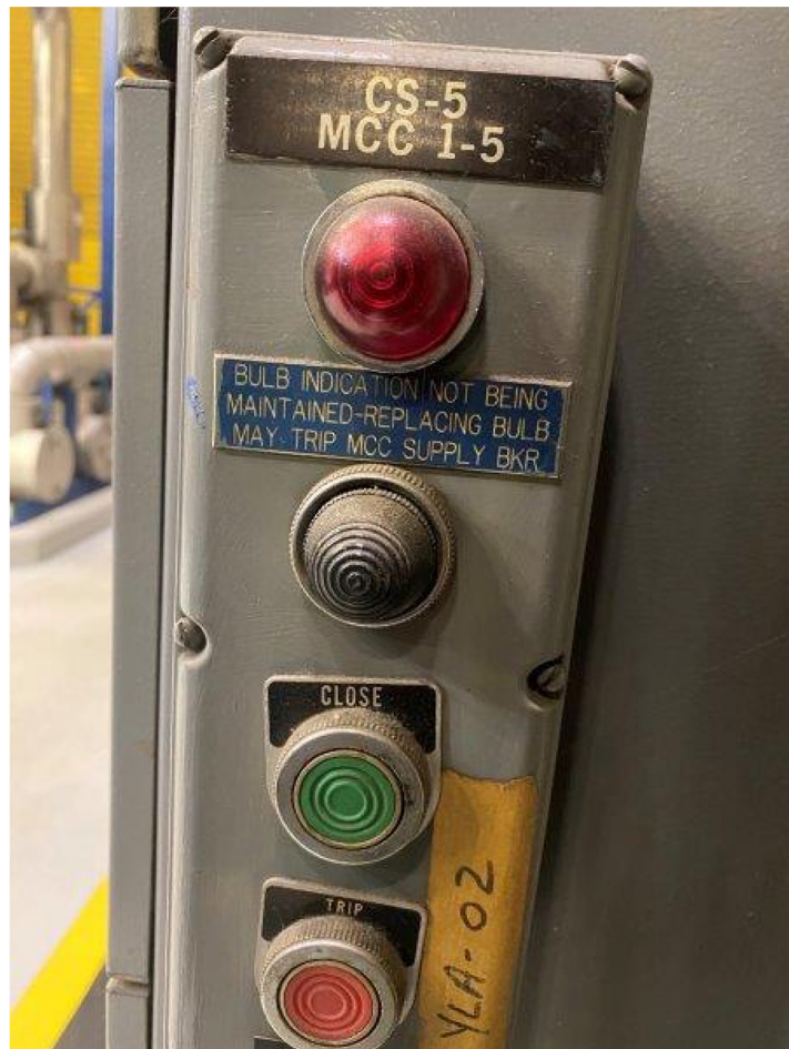
Figure 2 – Warning sign on equipment controls
