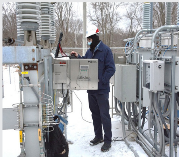
Figure 2. EPRI 138 kV research substation with some of the on-line monitors shown.
