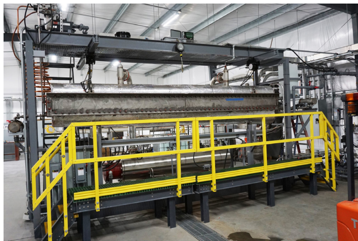
Figure 2. EPRI Water Testing and Conservation Center: Heat Exchanger Loop
