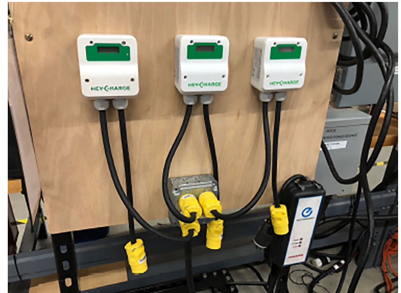
At EPRI’s EV laboratory, three HeyCharge access points with Bluetooth capability were deployed and tested for app-based, end-to-end management of the EV charging process.
