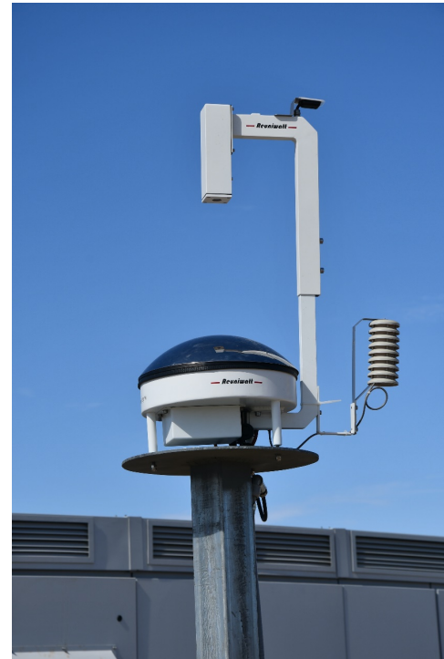
Figure 1-4 Photograph of Reuniwatt sky camera installed as part of short-term forecast service
