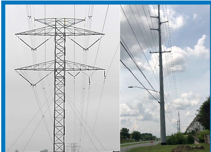
Figure 5: 400+132kV multi-circuit configuration, and multi-use structure supporting 138kV, 11kV under-build, telecoms, and streetlighting
