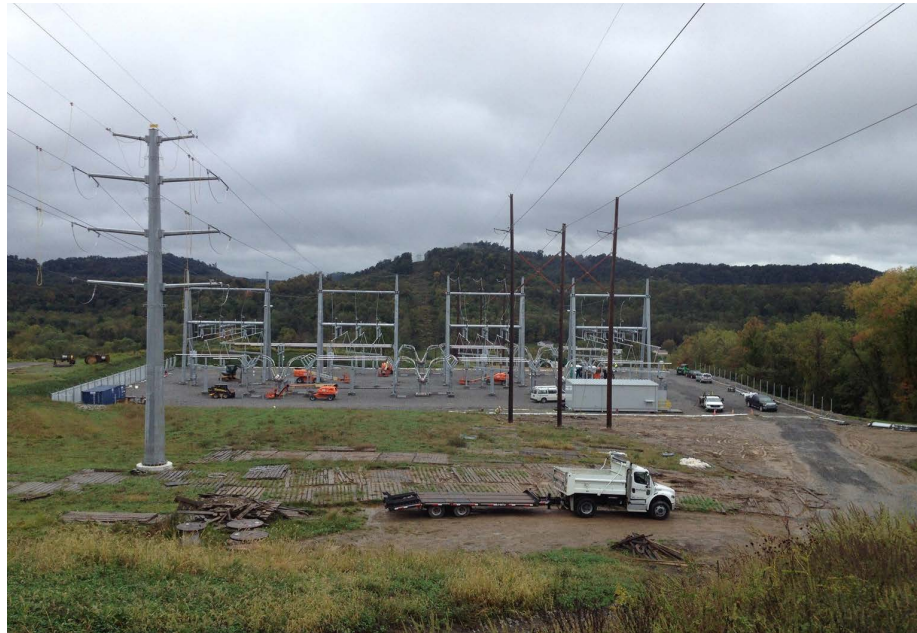
Figure 3-2 Substation near West Milford, WV. Credit: FirstEnergy Corp., Flickr.
