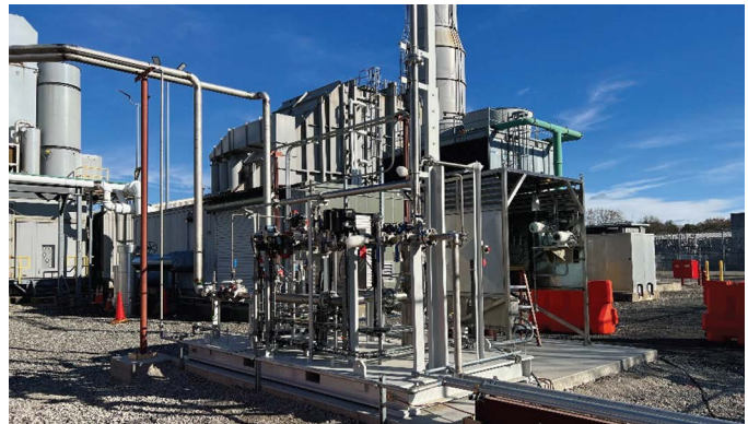
Figure 4. Hydrogen blending system and gas analyzer.
