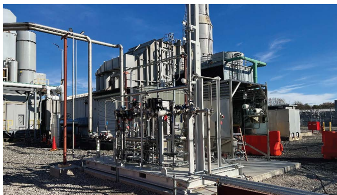
Figure 4. Hydrogen blending system and gas analyzer.
