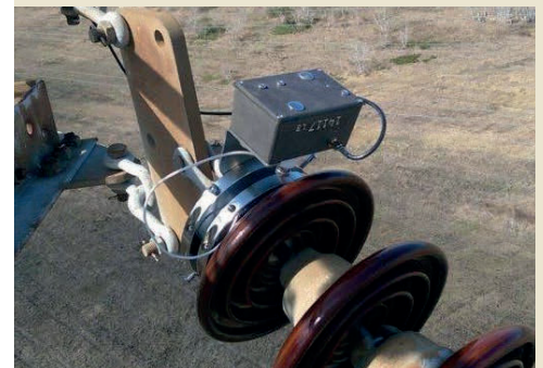
A suite of RF sensors have been developed for overhead transmission and substation applications. This is an example of a Clamp-on leakage current sensor installed on a porcelain disc insulator.
