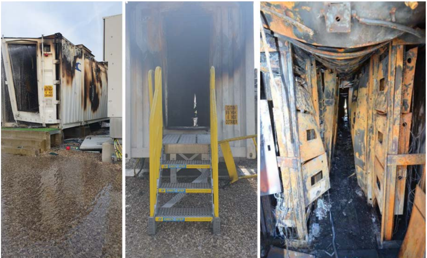
Figure 4 Image of doors blown open (source: NEC) and inside the container; source: MFRS
