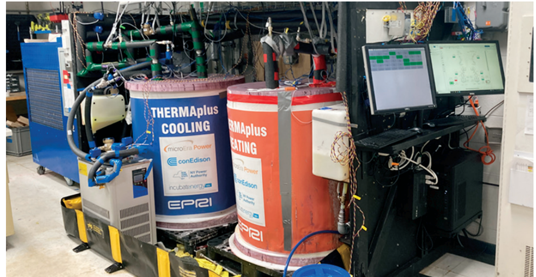
Insulated Tanks for Stored Cooling and Stored Heat, in MicroEra Power's Lab in Rochester, NY
