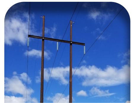
Ratings risk tends to be more important at lower voltages, e.g., these 115kV lines will overload rapidly if a 500kV line goes out.
