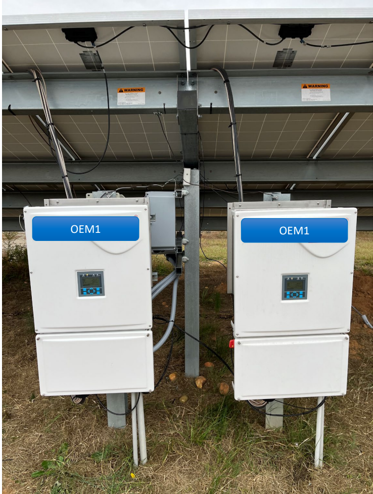
OEM1 inverter pair retrofitted with additional sensors and data monitoring box
