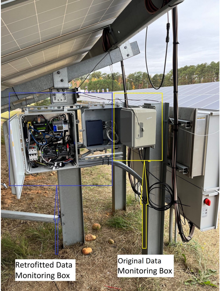
Retrofitted data monitoring box and original data monitoring box
