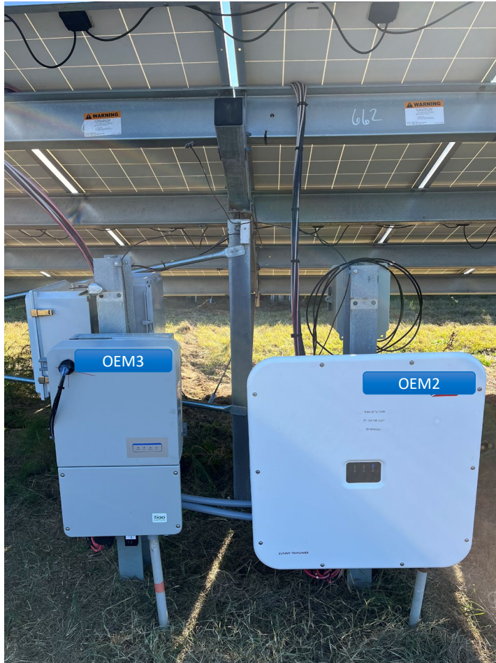
Instrumented inverter (SMA and Solectria) pair retrofitted with data acquisition box
