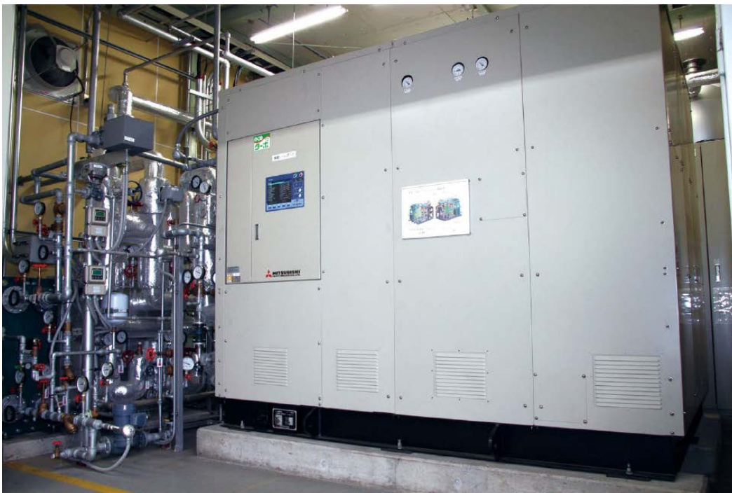
Figure 5. Mitsubishi Heavy Industries Heat Pump used at Takaoka Toko Oyama (Annex 58)
