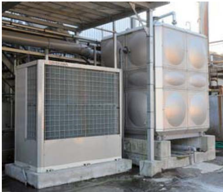
Figure 7. Mayekawa Eco-Cute Heat Pump and Thermal Storage Tank at Zennoh Kagoshima Oyama (JEHC)
