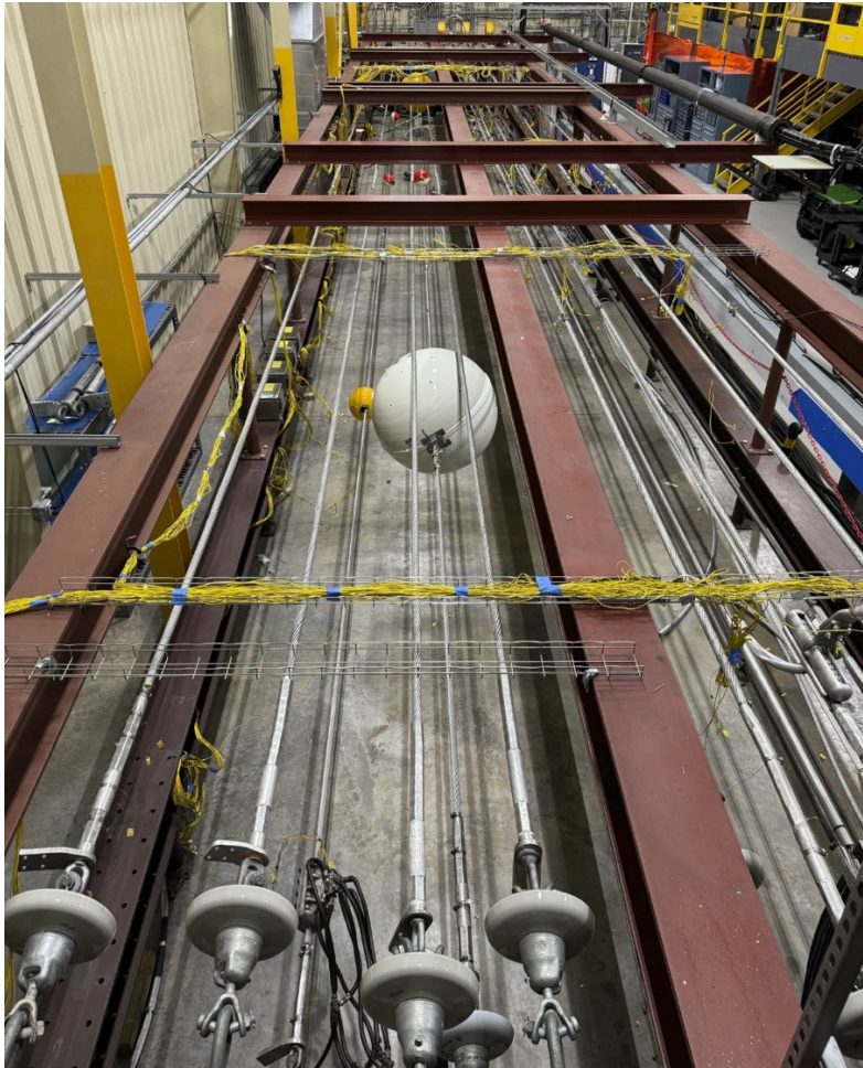
Figure 1. EPRI Charlotte, Conductor Test Bay
