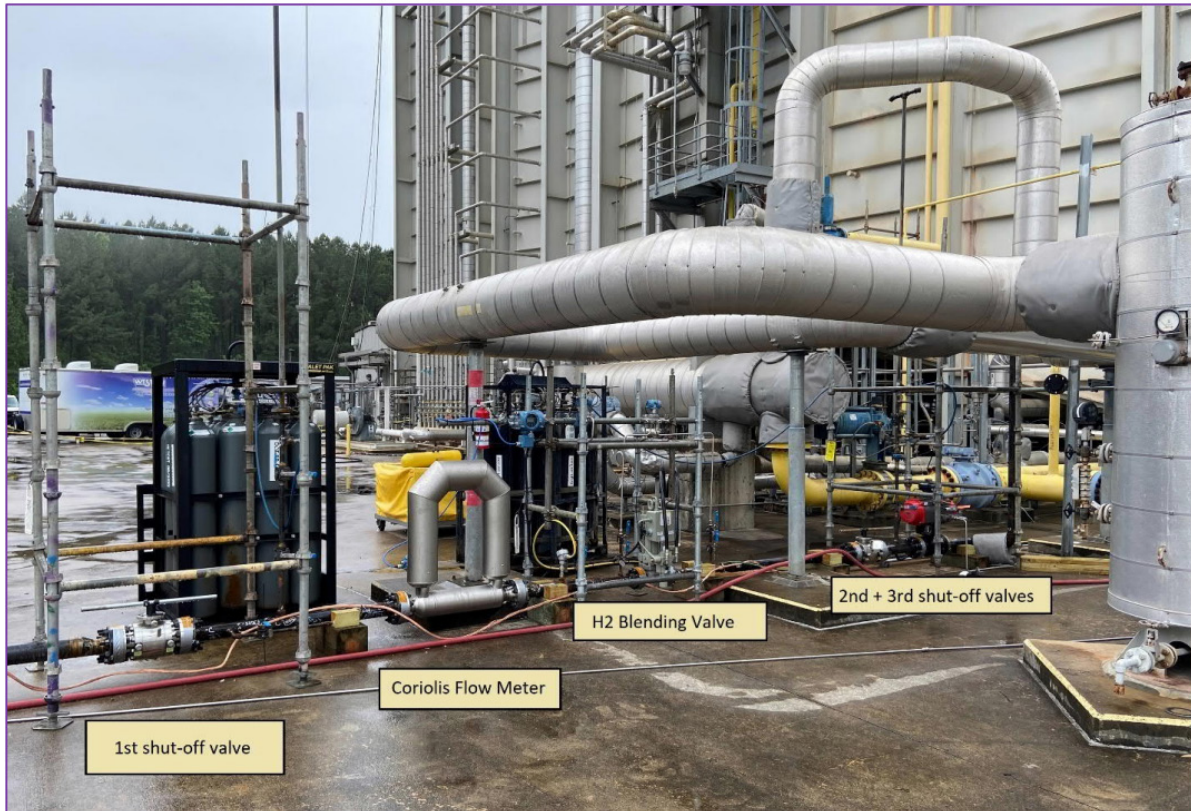
Figure 4. Hydrogen flow control system
