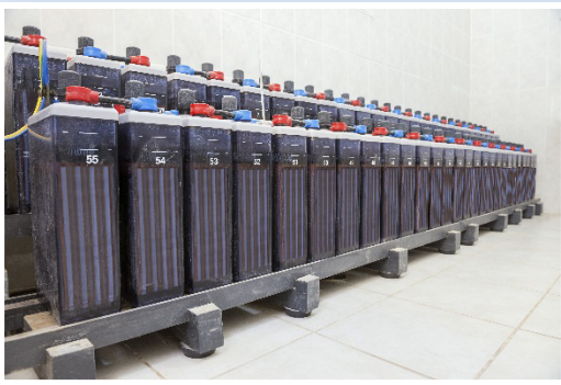
This project seeks to explore the performance of LiFePO4 batteries in substation applications
