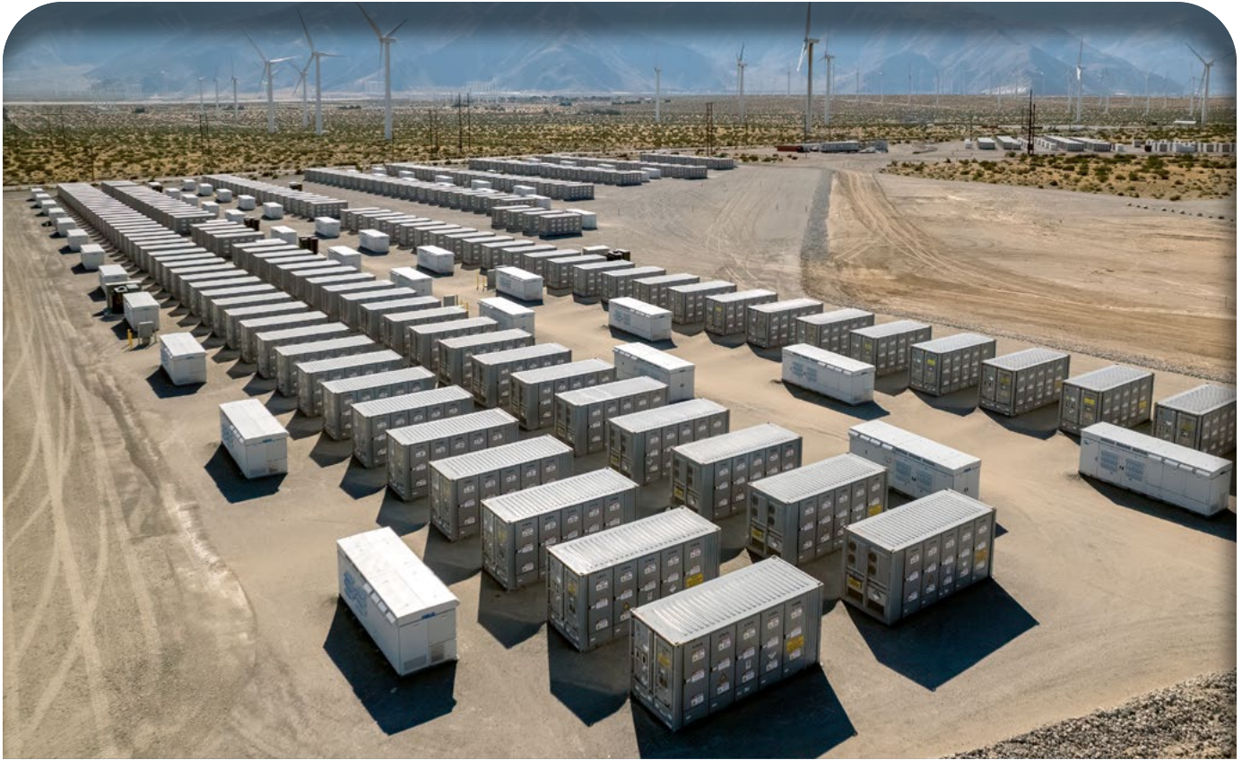
Figure 4. Current BESS facility designs typically include minimum separation distances between containers for batteries and ancillary equipment, as well as myriad other safety features.
