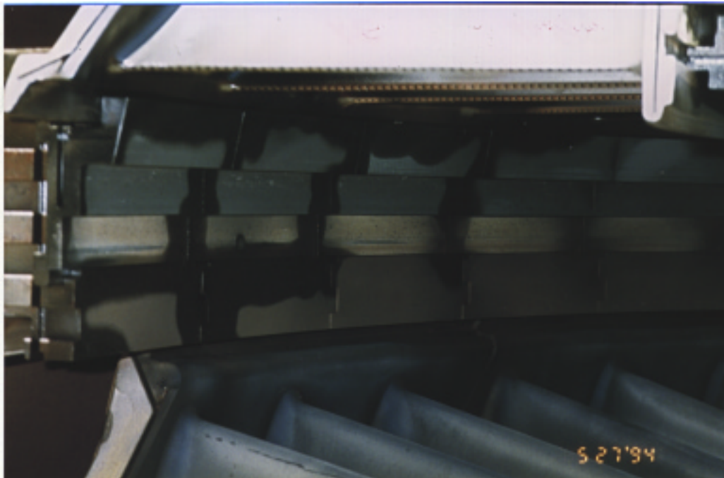
The 2nd stage stationary shroud appears to be in good condition. This is typical of others examined at the site.
