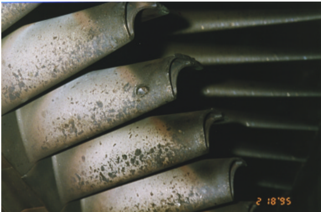
1st stage buckets showing convex side damage from compressor blade impactions. Figure 8.10 Unit 4A 2/95, 6,120 hrs. 1st Stage Buckets.
