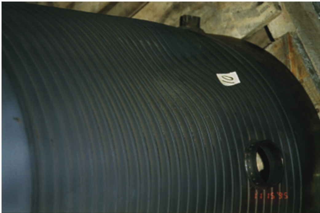
The combustion liner shows typical inward bulging distortion after 9,682 hours of operation. (seen on all liners.)
