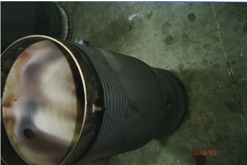
The combustion liner shows an inward bulging distortion after 8,504 hours of operation. Figure 8.42 Unit 3B 6/95, 12,586 hrs. Combustion Liner.
