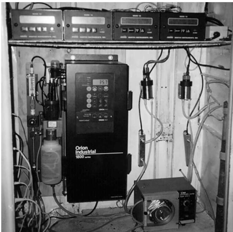
Figure 2-8 A View of On-Line Analyzers of the Inlet Steam Sampling System
