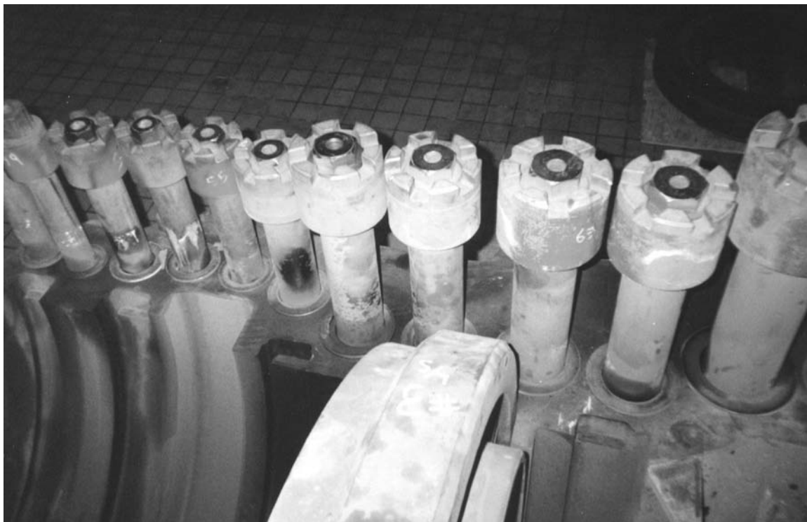
Figure 6-1 Photograph of HP turbine inner cylinder studs at Plant A.
